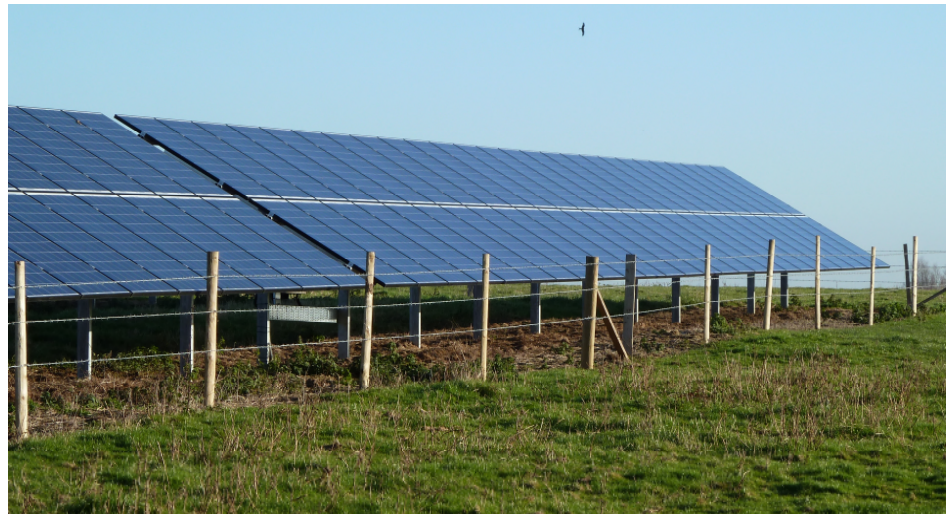
Solar PV Panels, Haddenham, Buckinghamshire, UK
